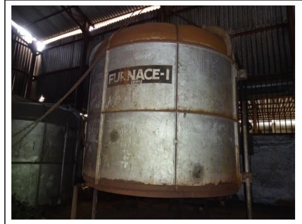
Fig. 3: Furnace for incineration
