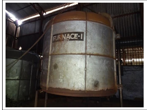
Fig. 3: Furnace for incineration
