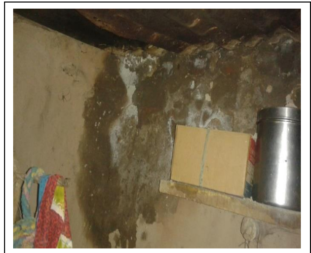
Fig.4: Leakage problems in earthen houses.
